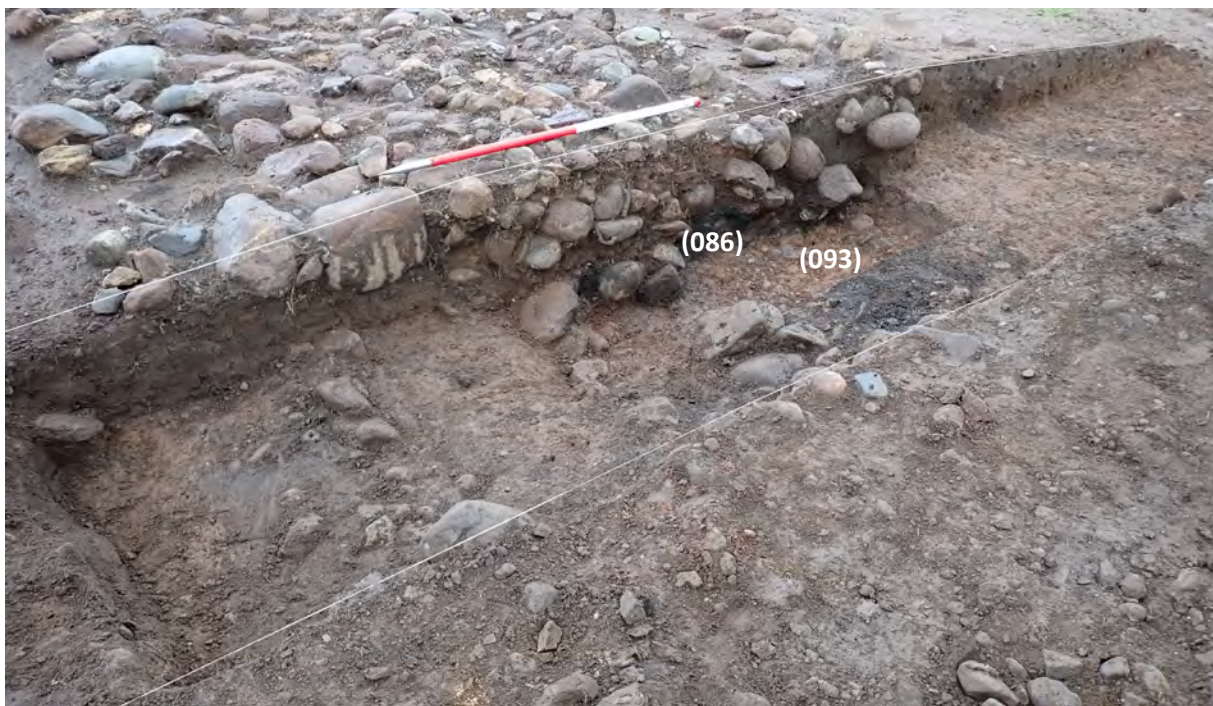
Figure 18: Slot 6 through road (003) showing construction trench (093) below with the industrial deposit (086), from north-east.
